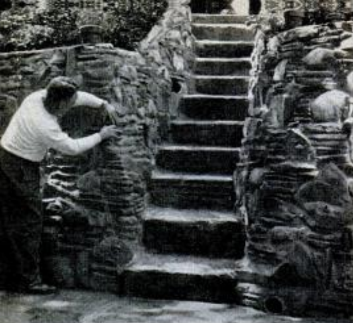
Wall of 2000 patterns was built around a terrace and steps. Each pattern consists of shale laid around a unique or colorful stone. Drainage holes keep wall dry
